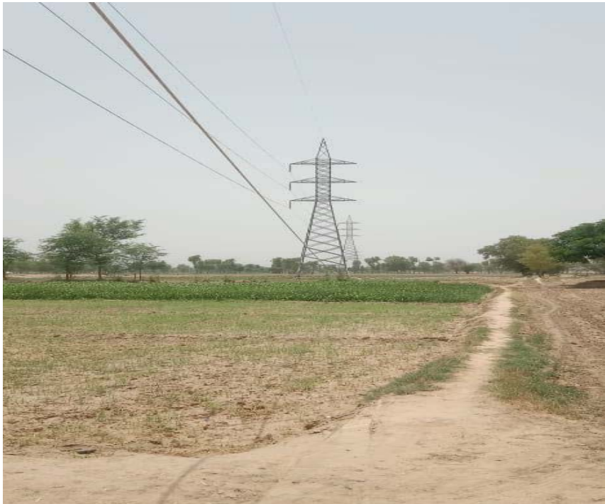
Newly Constructed 132KV Transmission Line 500KV RYK Sardar Garh to 132KV Feroza.
