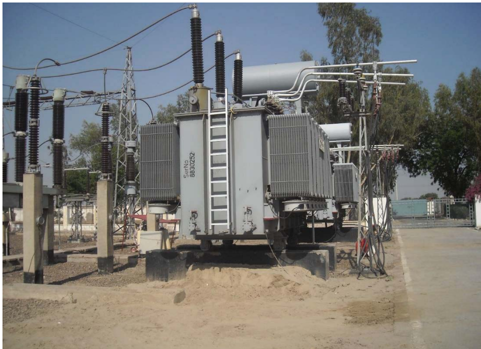
132 KV Grid Station Kacha Khu
