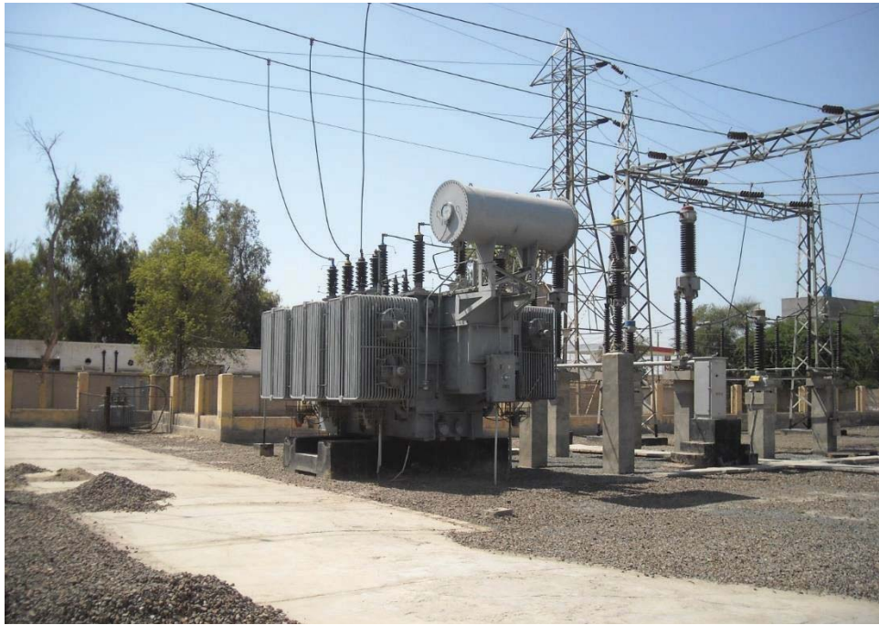
132Kv Grid Station Hasilpur
